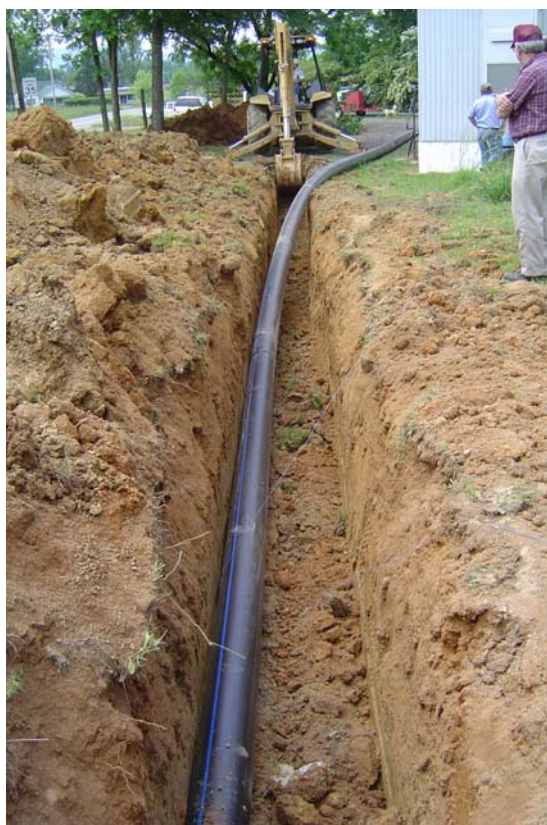
Polyethylene pipe is installed as part of a recently completed expansion of the Tri County water district in Yell County.
